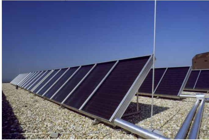
FIGURE 6. ARRANGEMENT OF PHOTOVOLTAIC PANELS FOR ALTERNATIVE ENERGY GENERATION IN BUILDINGS (SOURCE: WWW.WAGNER-SOLAR.COM)
