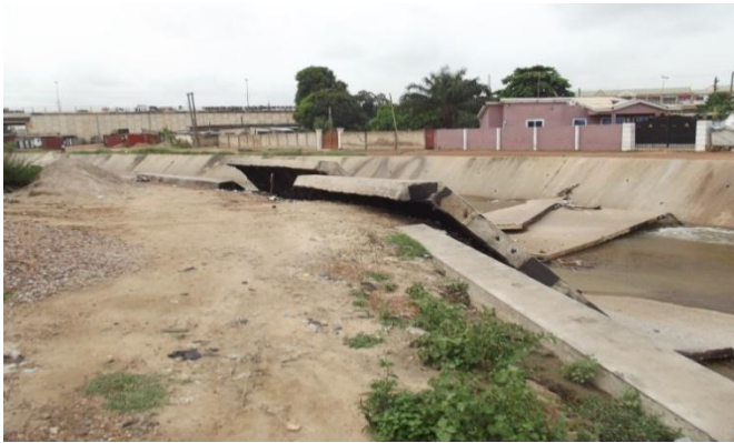
FIGURE 3 - IMPACT OF LARGE VOLUME FAST MOVING STORMWATER RUNOFF ON A STORM DRAIN IN ACCRA. Source: Author
