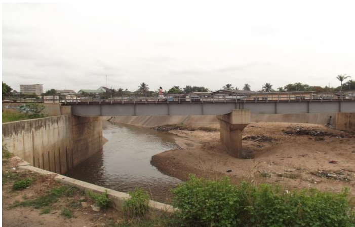
FIGURE 5 - SEDIMENTATION IN A SECTION OF A STORMWATER DRAIN IN ACCRA, GHANA. Source: Author
